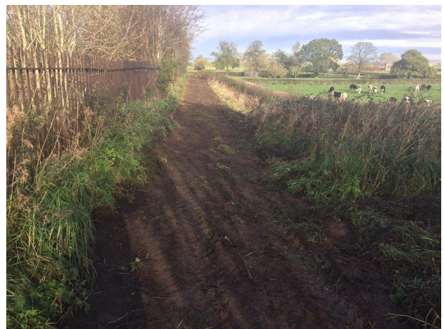
Work in progress to improve the footpath on the Wetlands (photo by Jayne Woollam).
