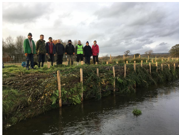
Brash bundles from the Wetlands used to prevent bank-side erosion of Bashall Brook (photo courtesy of Ribble Rivers Trust).
