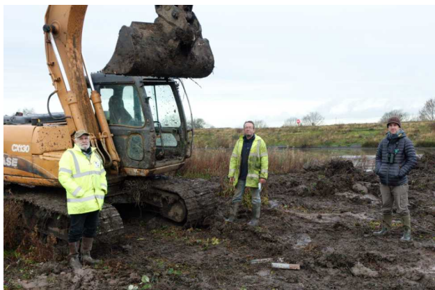
Project leader Geoff Carefoot (left), contractor John Dewhurst (centre) and consultant Gavin Thomas [RSPB Ecologist] (right) during a break from the island re-profiling work.
