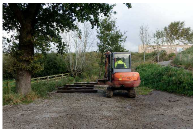
Contractor John Dewhust preparing the site for the installation of the storage container.
